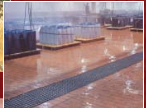
Carbo-Korez® floor in battery plant
