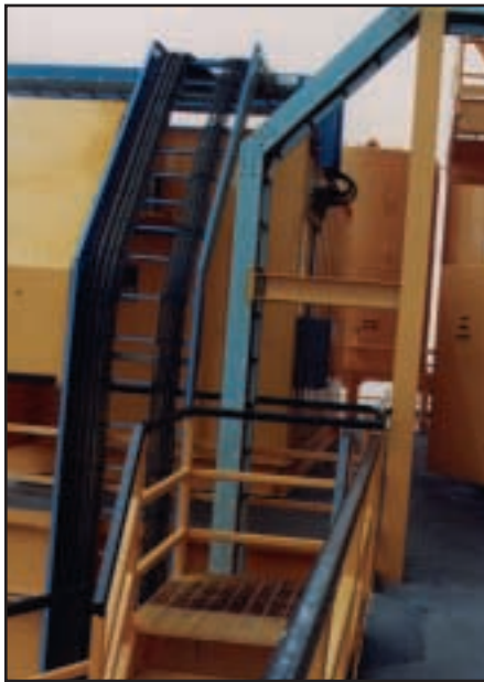
Vertical cable dropout from horizontal run
